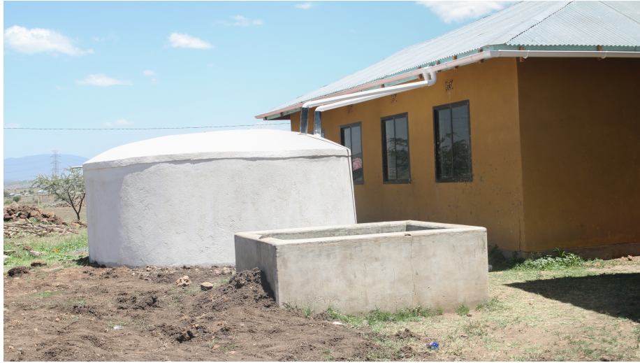
Figure 5: Water Harvesting Unit of 40k Litres [completed Feb 2023]
